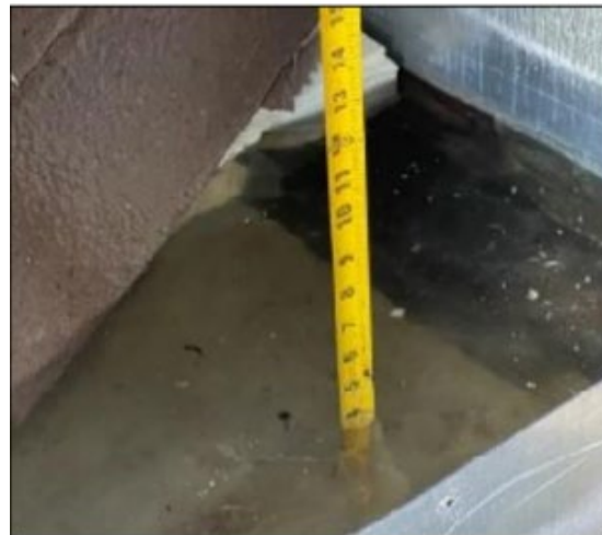
4. Standing water within dehumidification unit measured at 3.5 inches.
