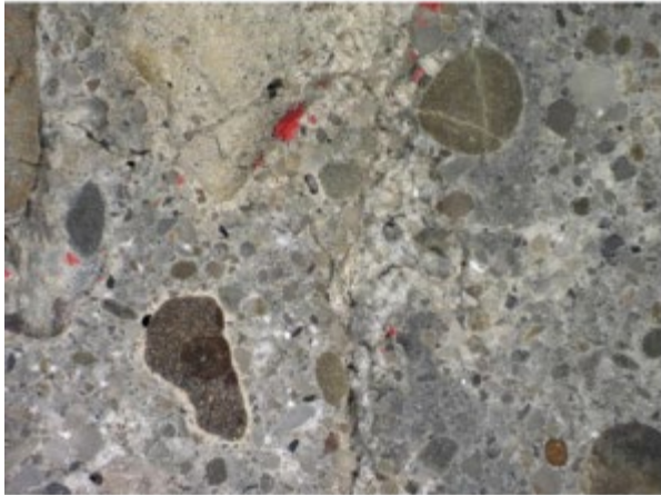
Photo 22: Core B-2 concrete with cracking near surface at suspected cold joint. 10x magnification.
