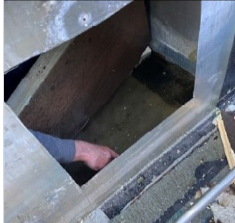
Standing water inside of dehumidification unit.
