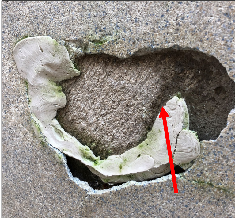
Plaster finish failed at a repair area.
