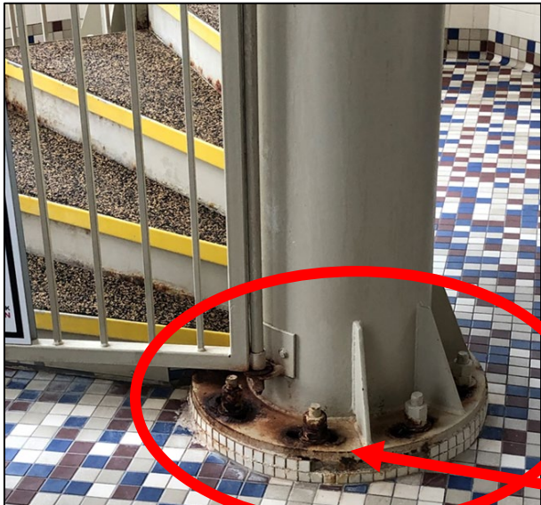
The slide platform is corroding.
