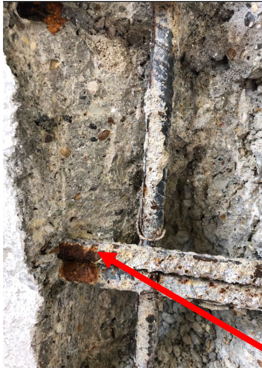
Moisture inside concrete rusting the metal (rebar) support system that holds pool walls upright.
