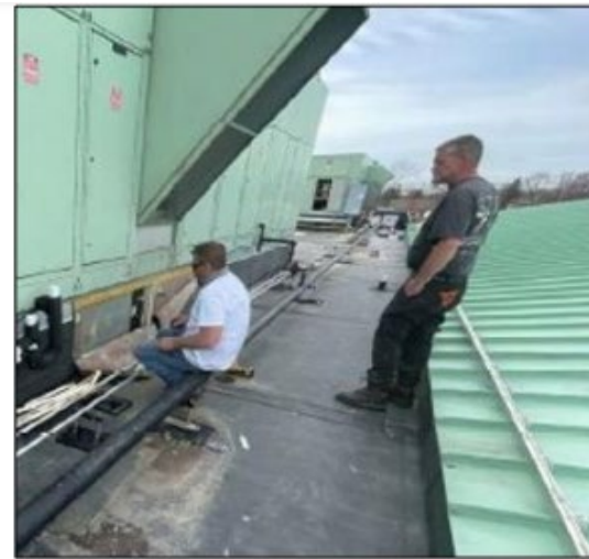
2. Hole cut into dehumidification unit to determine conditions within unit.
