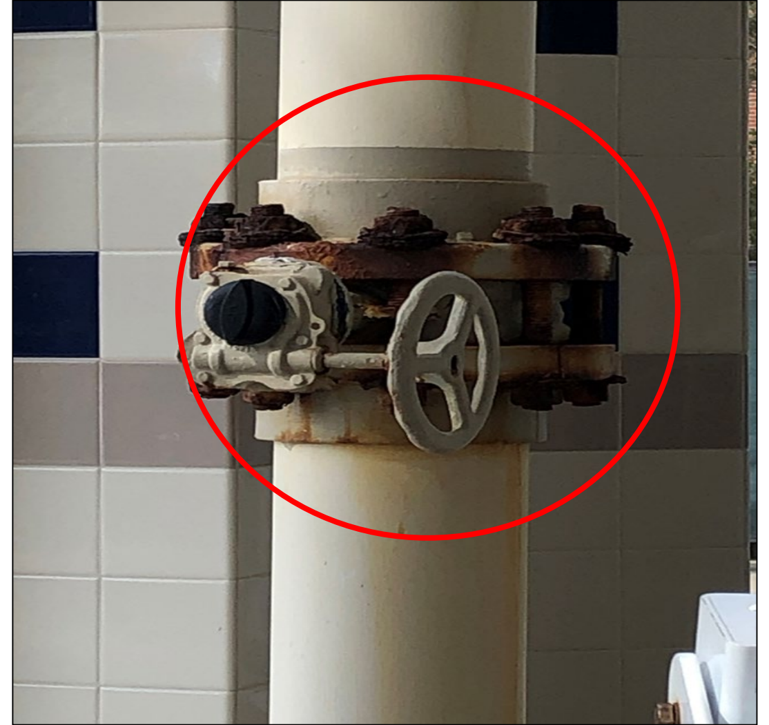
Water feature valve is rusting and deteriorating.
