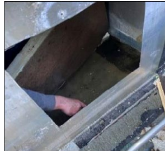
5. Contractor observes standing water inside of dehumidification unit.
