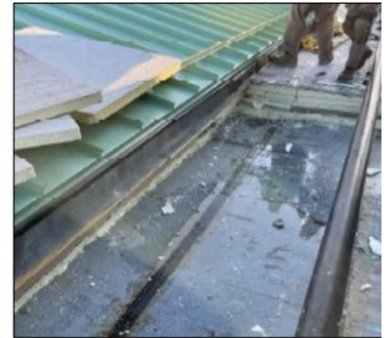
6. Roofing material removed near dehumidification unit, revealing standing water within roofing system.
