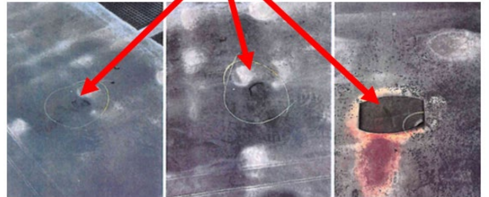
Previous repairs failing
