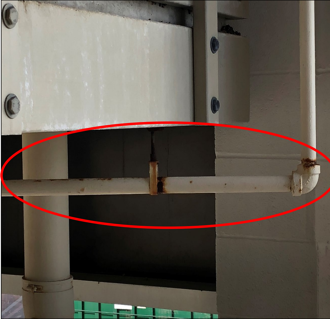
Fire suppression system is rusting and deteriorating.
