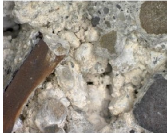
Photo 25: Core B-3 concrete at steel reinforcement 9-inches deep with consolidation void. 10x magnification.
